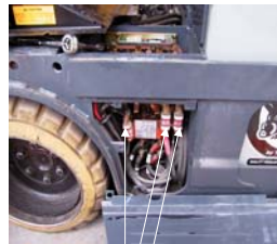
Main truck fuses are located on the contactor panel assembly
