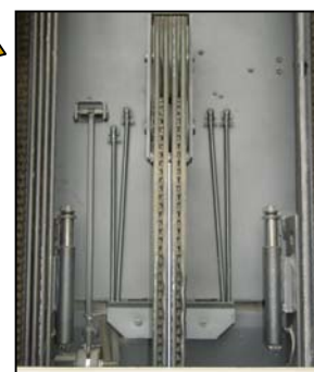
Crown control system and traction motor. Crown chassis to platform cabling
