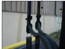
Metal tension spring clips used on electrical cables
